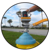
Hydrant Key Available
